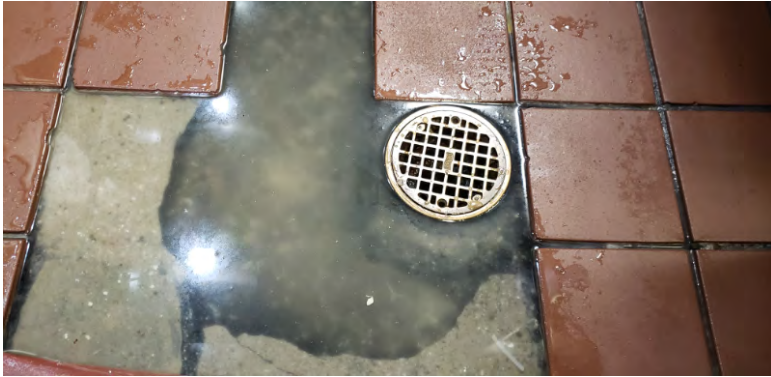
Water pooling around floor drain
